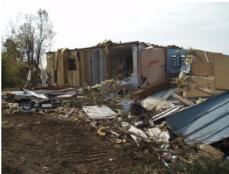
This building north of Paris, TN was badly damaged by thunderstorm winds on November 6th.
