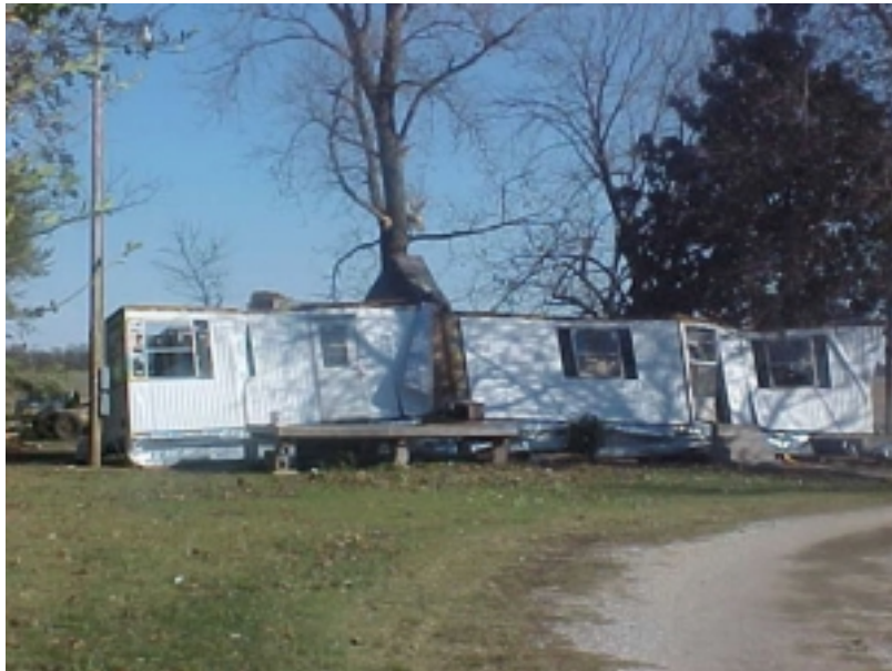
This mobile home in Lawrence County was damaged by thunderstorm winds on November 15th.
