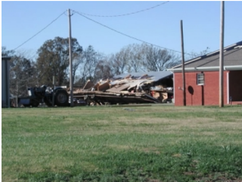
This mobile home in Gibson County was badly damaged by a tornado on November 15th.
