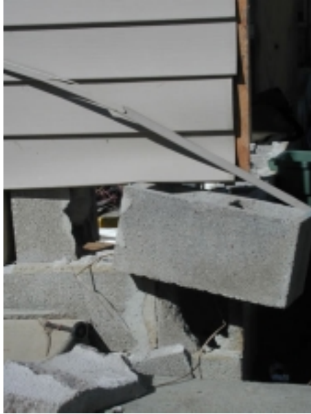
This house in Crockett County was shifted off its foundation by a tornado on November 15th.
