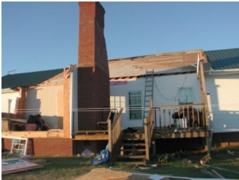
This home in Weakley County was damaged by a tornado on November 15th.
